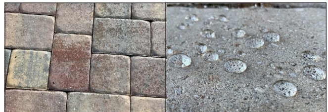
Surfaces requiring to be stripped
