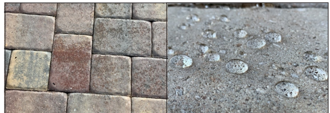
Surfaces requiring to be stripped
